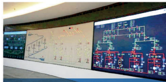
南方电网清远蓄能电站计算机监控系统 CSCS of Qingyuan pump storage power station, China Southern Power Grid
