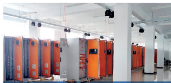
计算机监控系统装配调试车间 Workshop for assembling and debugging of CSCS
